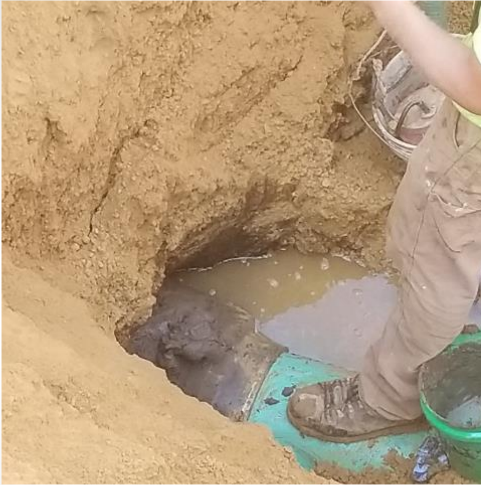
Existing sanitary sewer is clay tile and in poor condition
