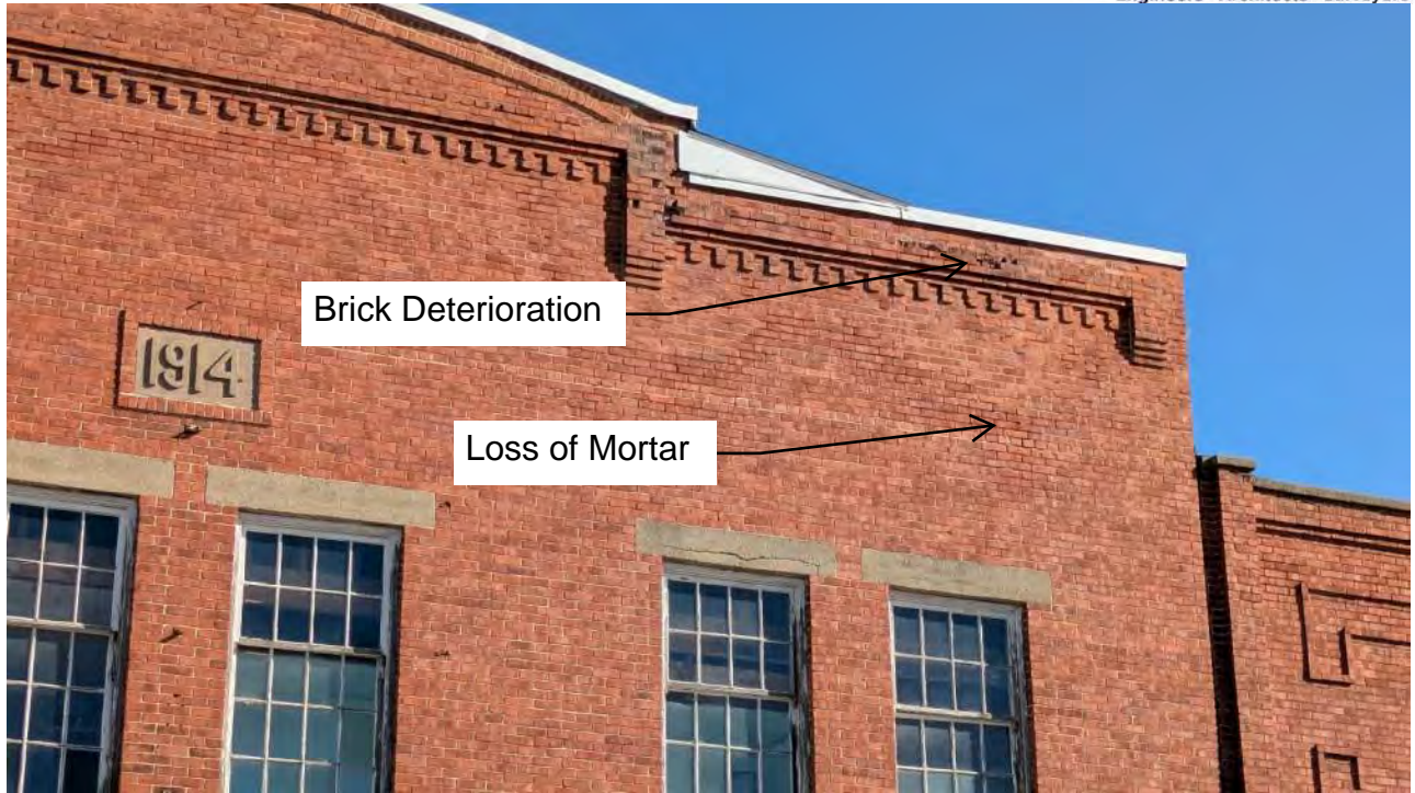
Photo 9 – Exterior, South wall, mortar missing in areas of exterior brick face
