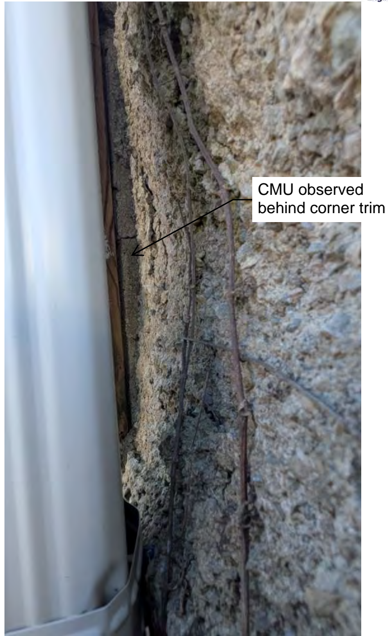
Photo 23 – Independent CMU wall observed behind corner trim at Northeast corner of 230 E Main Street
