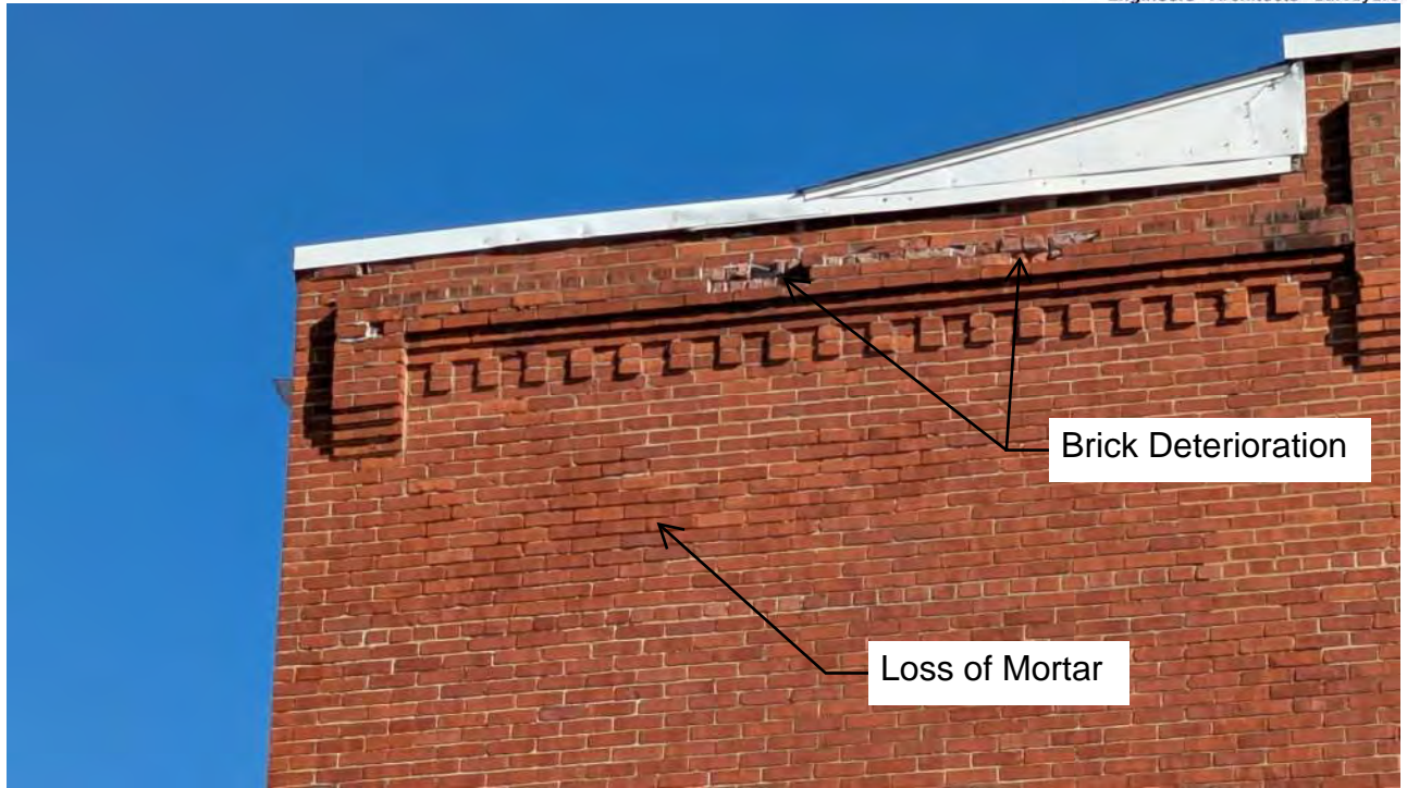
Photo 11 – Exterior, South wall, mortar missing in areas of exterior brick face
