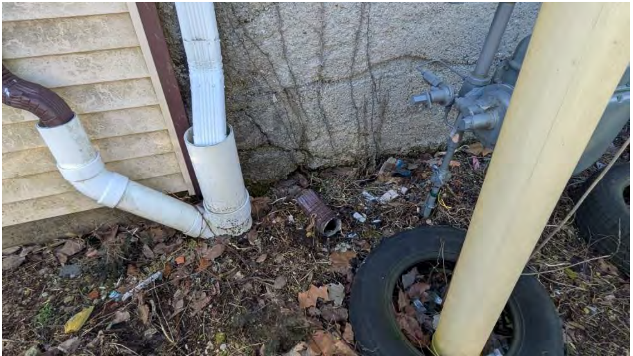
Photo 22 – Concrete wall deterioration at Northeast corner of 230 E Main Street
