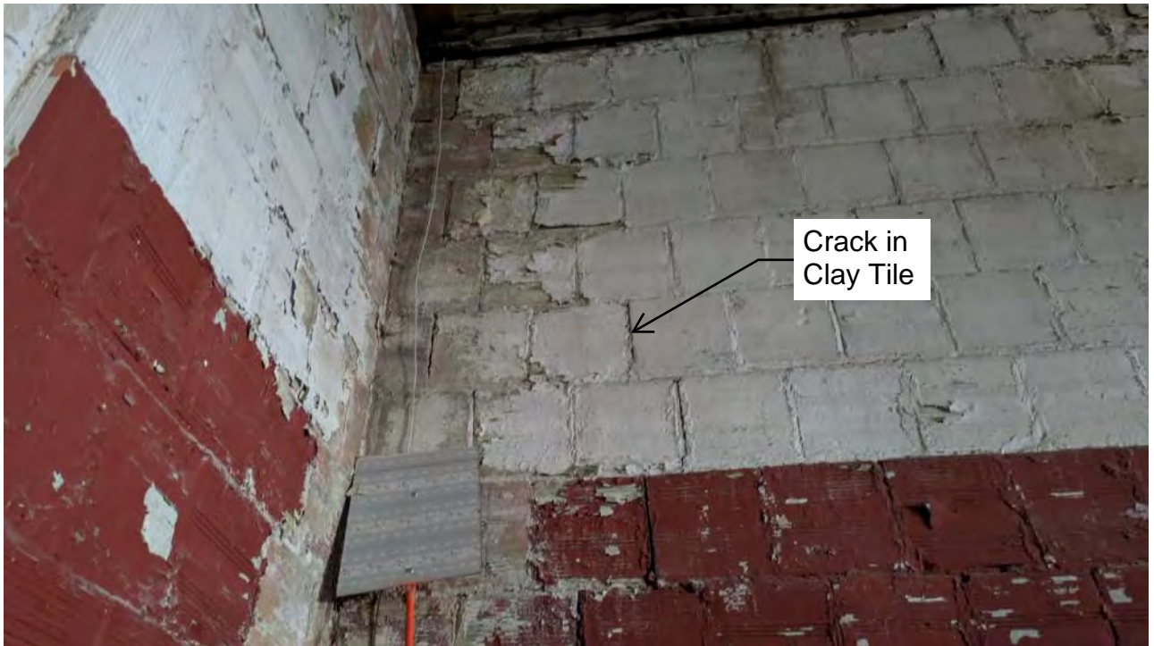
Photo 6 – Upper Level, vertical crack in clay tile wall, Northeast corner
