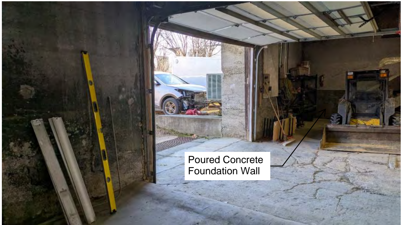
Photo 8 – Basement Level, Overhead door in North wall, East wall is poured concrete
