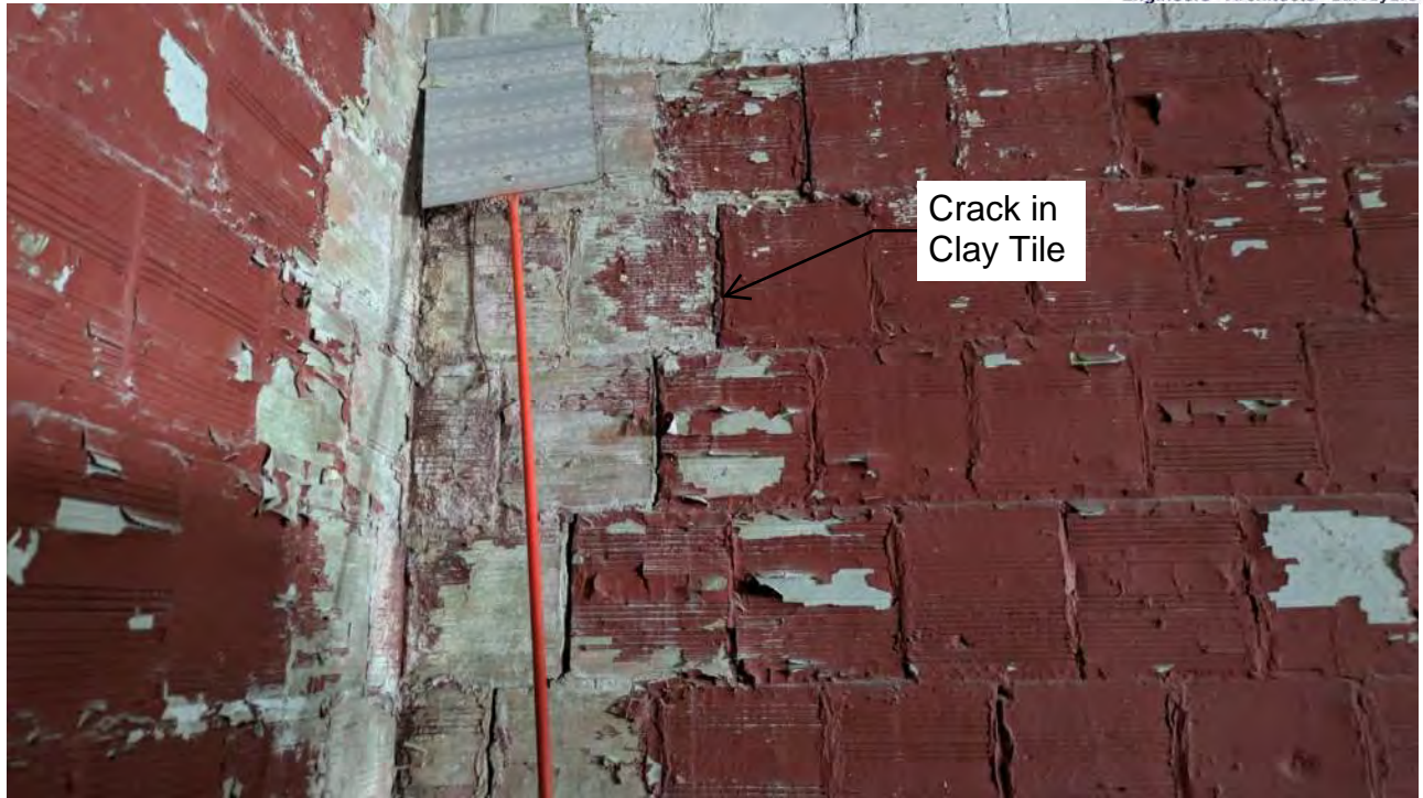
Photo 7 – Upper Level, vertical crack in clay tile wall, Northeast corner
