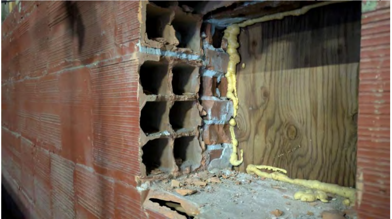
Photo 5 – Upper Level, knock-out in North wall. Clay tile, air space, clay brick
