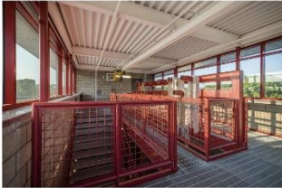
UPPER PLATFORM: HOSE DRYING, STANDPIPE, ROOF ACCESS
