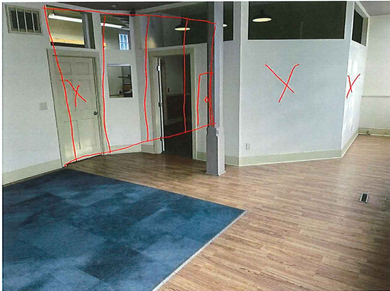
Figure 8: Walls to be removed and door will shift to the right limits of the new wall
