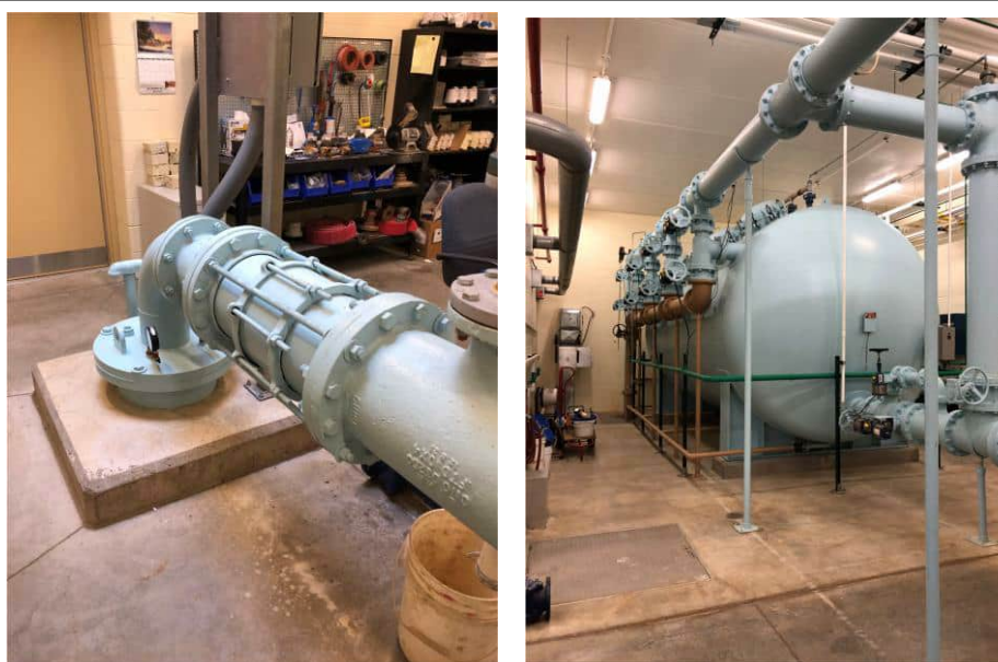
Figure 2.02-3 Well No. 5 Well Head and Filter System
